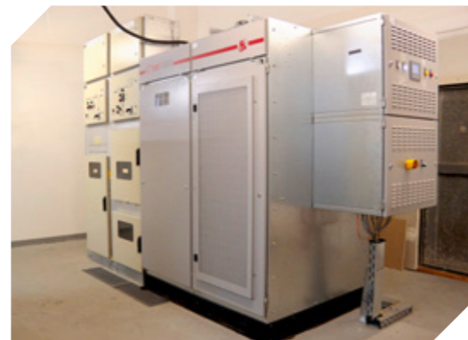
The soft-starter developed especially for VEM to enable the stress-free starting and synchronisation of 10 MVA synchronous-synchronous railway converters. Photo: F&S PROZESSAUTOMATION GmbH
