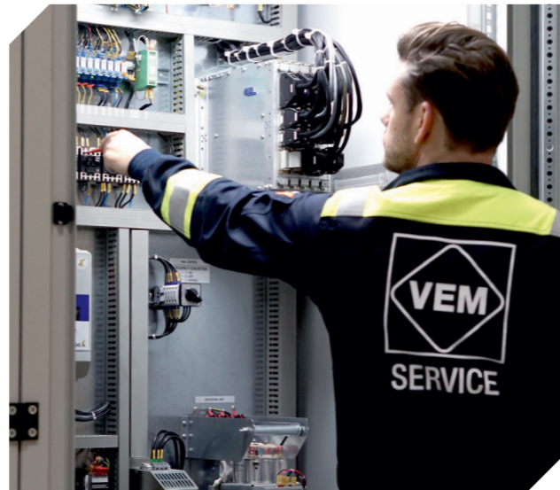
The customer can continue to use the existing motors and pumps with the new reliable technology and modern plant control.
