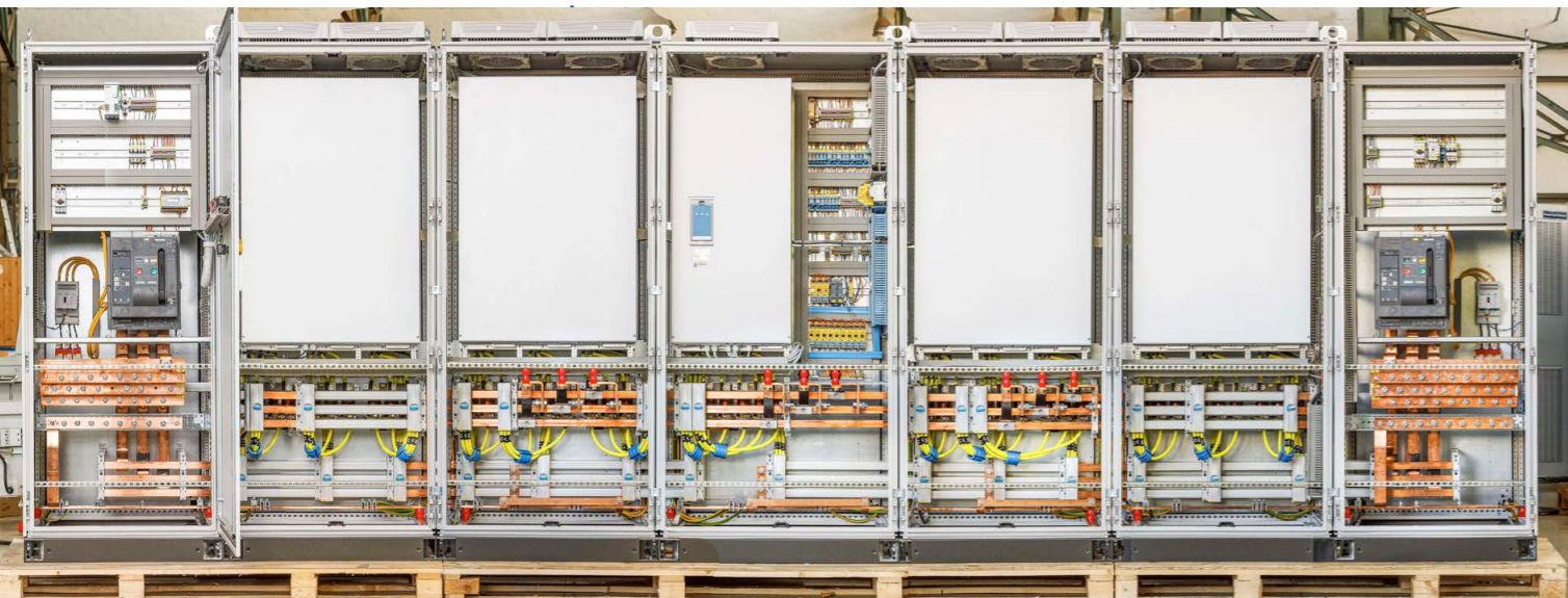
The new converter which has already been installed by VEM
