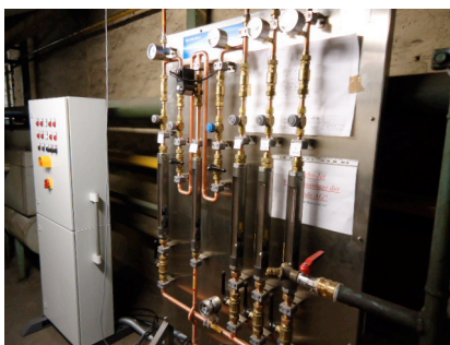
Test installation of the Carbojet® gas control panels for setting of the nitrogen and hydrogen flow rates
